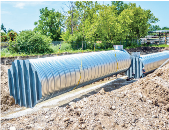
CORRUGATED STEEL PIPE (CSP)
