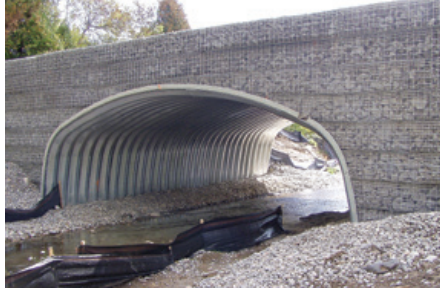
ROCK FACE WIRE MESH WITH MECHANICALLY STABILIZED EARTH (MSE) RETAINING WALLS
