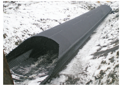
MINISTÈRE DES TRANSPORTS / MINISTRY TRANSPORTATION QUÉBEC (MTQ) - MULTI-PLATE PIPE-ARCH WITH STRATA-CAT COATING
