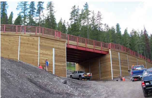
WOOD FACING ENHANCES THE NATURAL APPEARANCE OF THIS BIN WALL BRIDGE ABUTMENT
